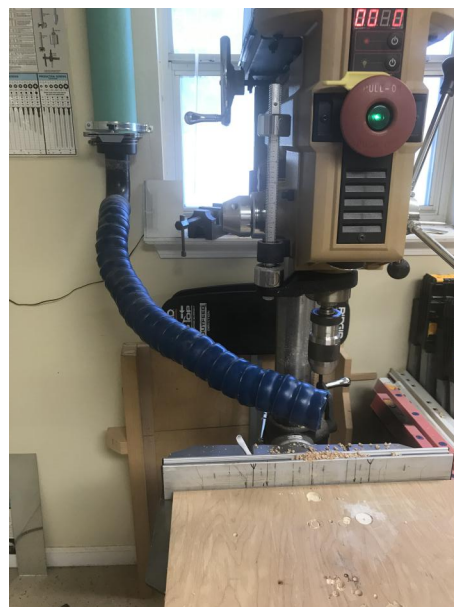
Tom Gustafson's dust collection system for the drill press. Semi-rigid loc-link hose connects to his four-inch line at one end and is positioned very close to the drill bit at the other end.
